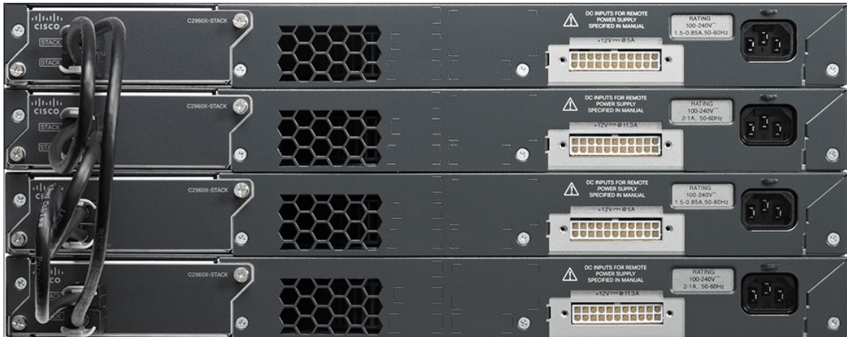
Figure 6-15 Photo of Four 2960X Switches Cabled on the Left with Stacking Cables
